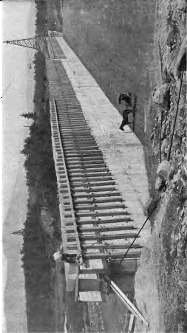
PLATE 47.—View of Core Wall for Beaverkill Dike, Cantilever Forms, and Cableway Used for Placing Concrete, etc.
